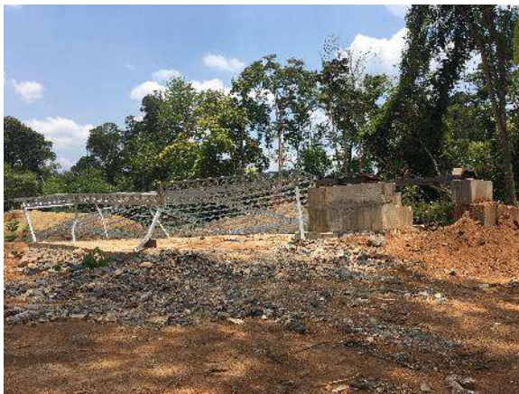
Incomplete (and now collapsed) metal frame building associated with new Chinese mine development.
