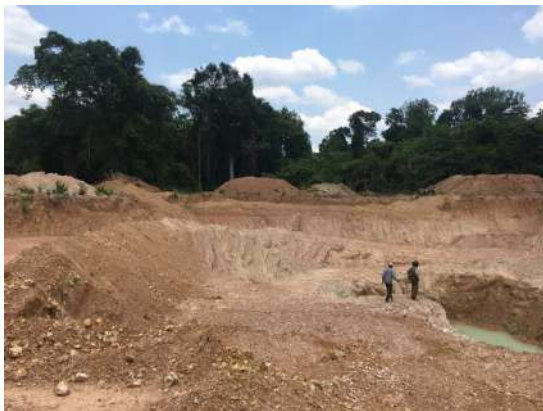
Large excavated open mining pit associated with new Chinese mine dev. (location marked with pentagon in Sec. 4a, Fig. 5.) This area is now the large open pit mine in the main mine.
