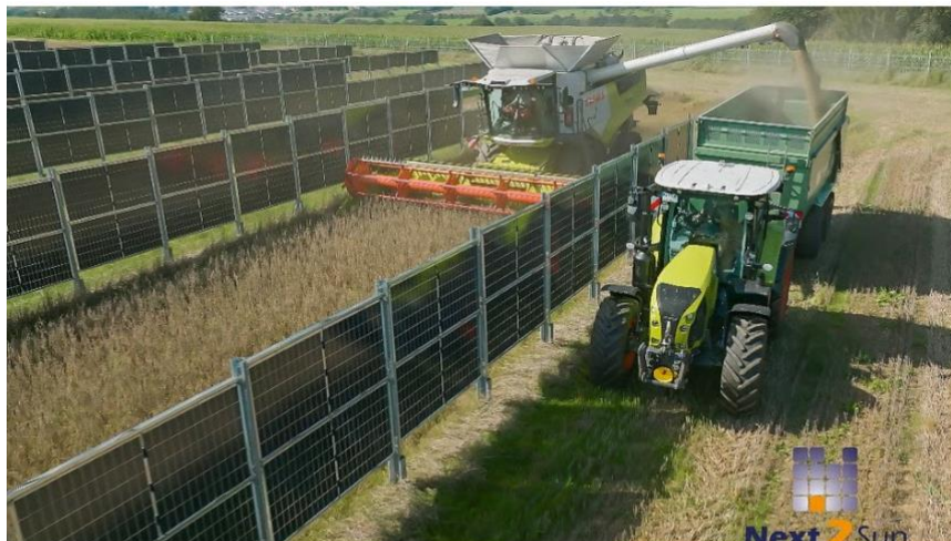
Next2Sun's 5.2 MW Agrivoltaic vertical PV installation, featuring Huasun's Kunlun series HJT module, exceeds power generation expectations by 12%, noted the project manager. (Photo Credit: Huasun)
